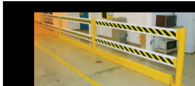
Incorporate multiple barrier systems to create a highly visible barrier for pedestrians and fork trucks.
