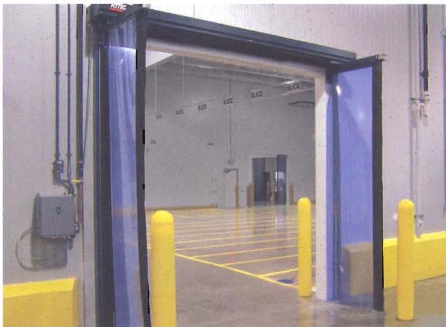
Photo courtesy of Rytec Corporation
